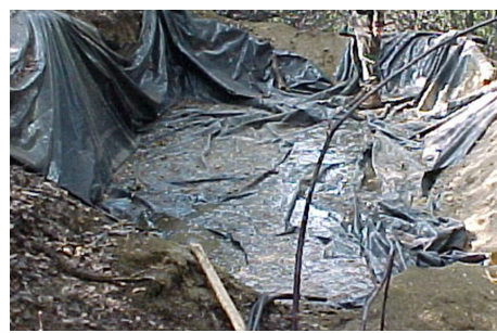
Water diversion cistern
