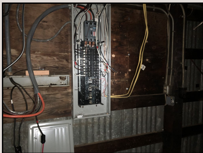
Glendale grow site electrical system
